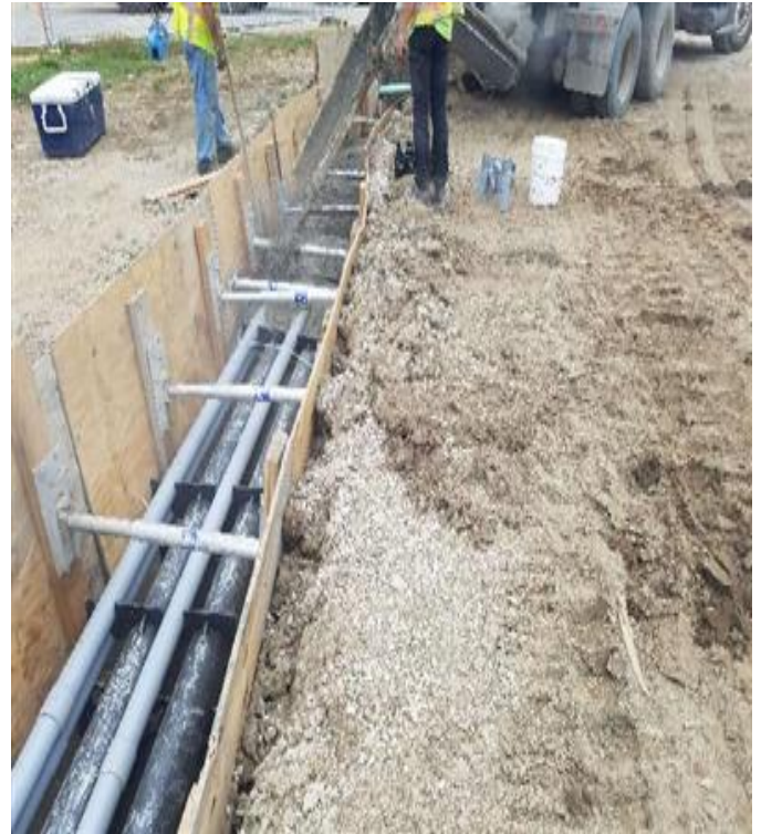
Fig 10: McCourt pouring concrete for duct bank in trench along Colovos road. Viewing north. (7-22-19).
