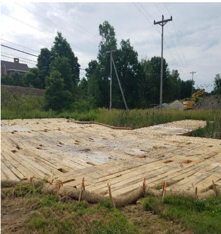
Fig 15: Timber matting for work pad, with BMP installation at Str. 24. Viewing southeast. (7-22-19).
