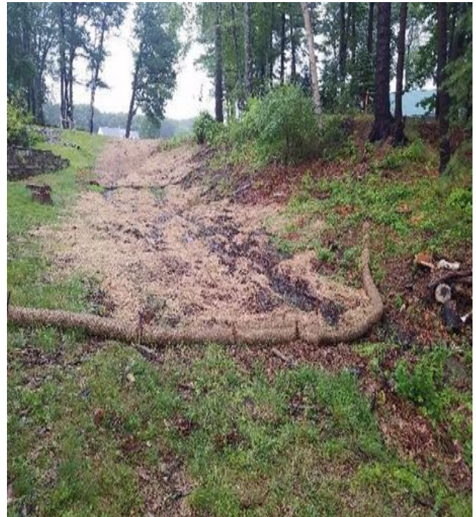
Fig 16: Gundalow Landing erosion controls, additional fence and bales are required. Viewing northeast. (7-23-19).
