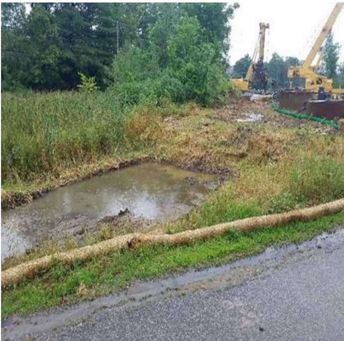
Fig 19: Wetland DW69, location of where straw bales need to be installed. Viewing east. (7-23-19).
