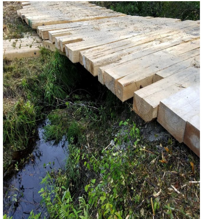
Fig 14: Downstream view on west side of temporary mat bridge over Stream DS60. Viewing north. (7-22-19).
